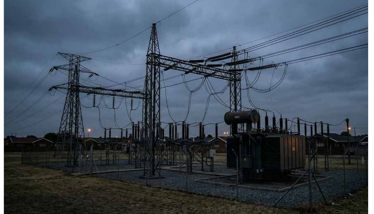
Protecting power infrastructure ... Emergency load rotation was implemented to protect infrastructure from damage because of bad weather. Picture: Facebook
