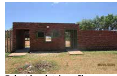
Dilapidated ticket office
